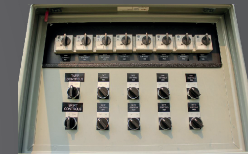
CONTROL PANEL for tarp and skirts
